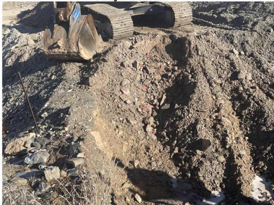
AOC14 TAA1 Visible debris with potential ACM - Facing North
