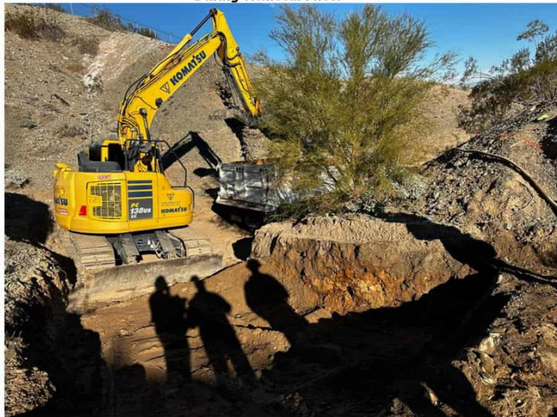
AOC10 TAA2 West end of excavation. Rust discoloration under Palo Verde tree - Facing Northeast
