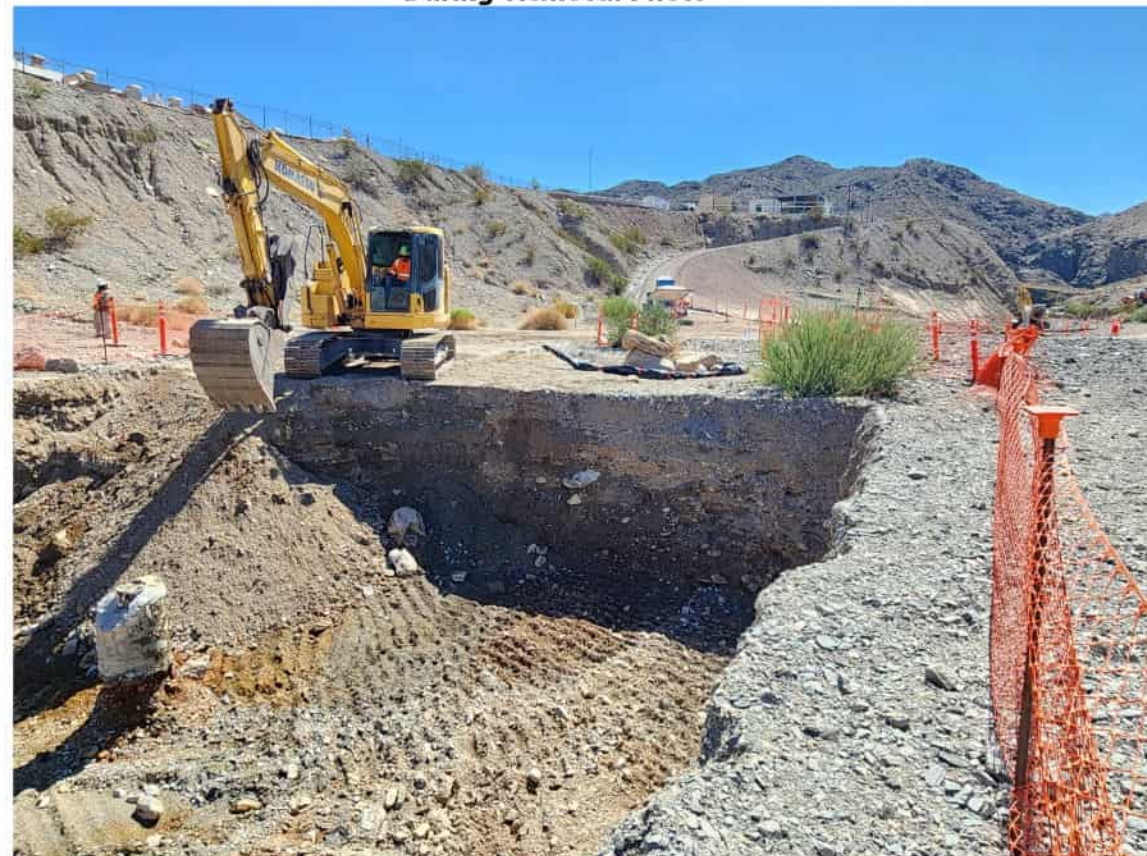
AOC1 TAA2 TCS-4 well uncovered and visible brownish orange discolored soil - Facing Southeast
