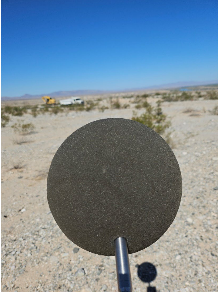
Photograph 2-5B. Noise Monitoring Location West of the Access Road to Bat Cave Wash, on Same Elevation as Topock Maze, Looking Northwest at NTCRA Construction Equipment Traffic
