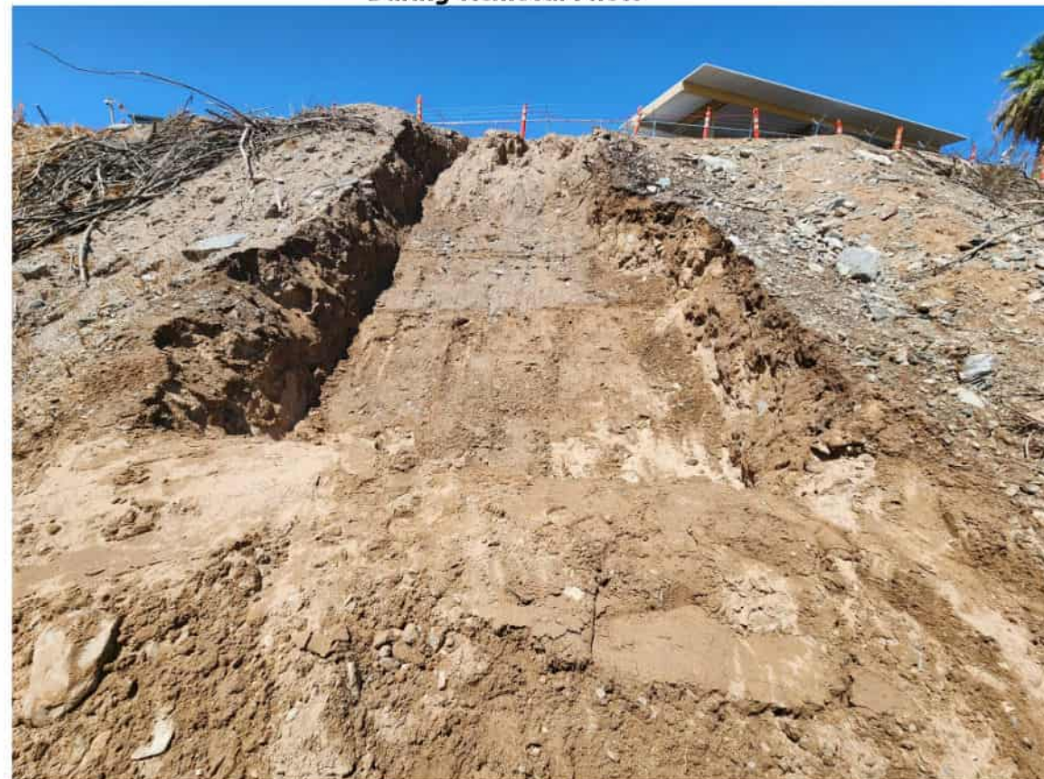
AOC10 TAA1 Visible white powder and rust discolored soil - Facing West
