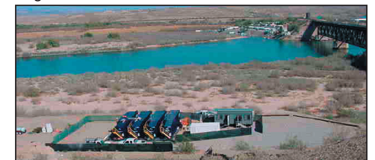
Interim Measures equipment, including water storage tanks
