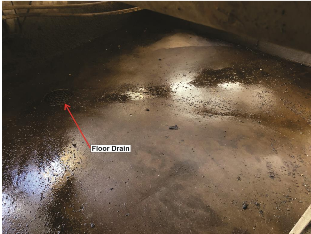
Photograph 4.2.21-3: June 14, 2022, Compressor Engine Basement.
