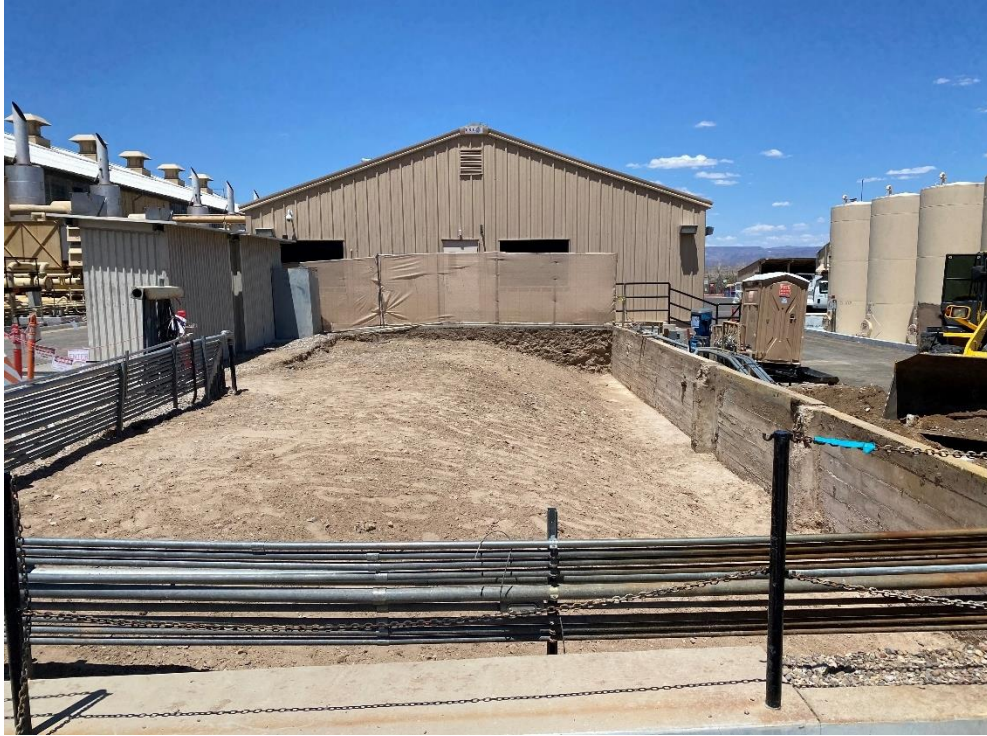
Photograph 4.2.11-3: August 2020 Photograph of the Completed Excavation Area at AOC 15. Note: Looking north.
