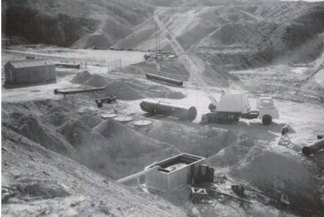
Photograph 4.2.20-3: January 26, 1954, Construction Photograph, Oil/Water Separator Installation Note: Facing southwest. Discharge line emanating from the OWS is visible in bottom right.
