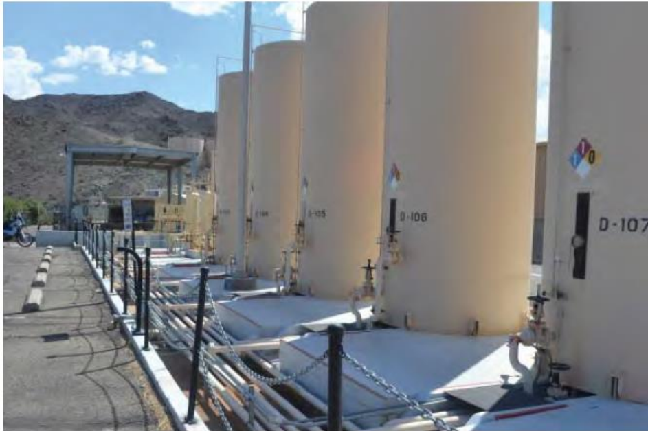
Photograph 4.2.23-4: August 21, 2012, Tanks, Containment, and Trench Notes: Facing south. Photo includes the pipe trench on the eastern side.
