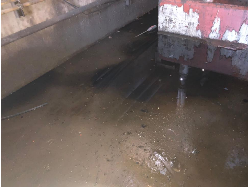
Photograph 4.2.21-7: June 14, 2022, Oil Staining and Accumulation in a Compressor Engine Basement.
