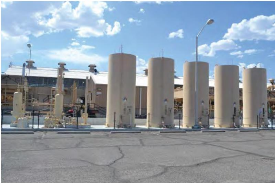
Photograph 4.2.23-3: August 21, 2012, Oil Storage Tanks and Concrete Containment Note: Facing west.
