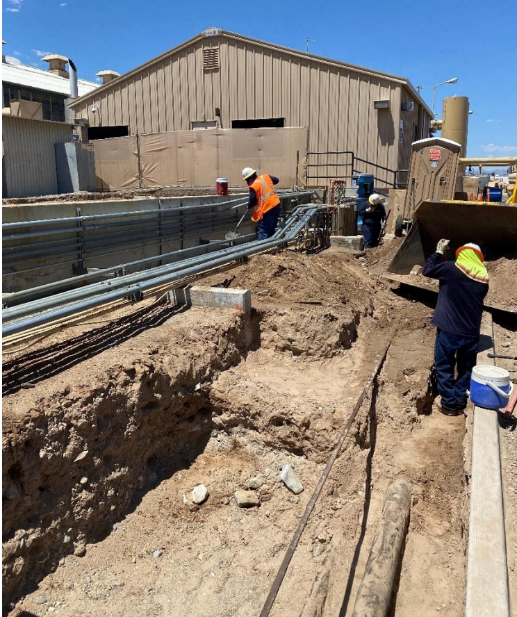
Photograph 4.2.11-2: August 2020 Photograph of the Excavation in Progress at AOC 15 Note: Looking north.
