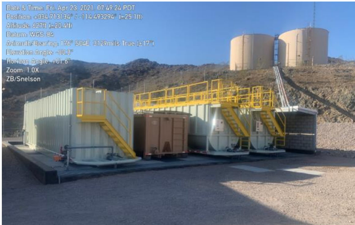
Photograph 4.2.8-2: April 23, 2021, Photograph of The Water Conditioning Tank Farm Note: Constructed over the former hazardous materials storage area. Photo facing south.
