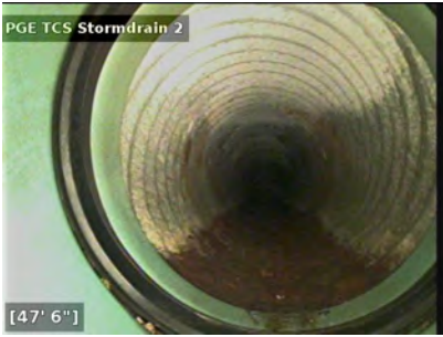
Transition from blue PVC to corrugated steel pipe.
