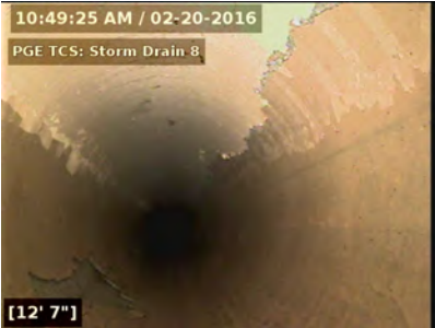
2/20/2016 10:49:26 AM Small cracks or scale in bottom of pipe.
