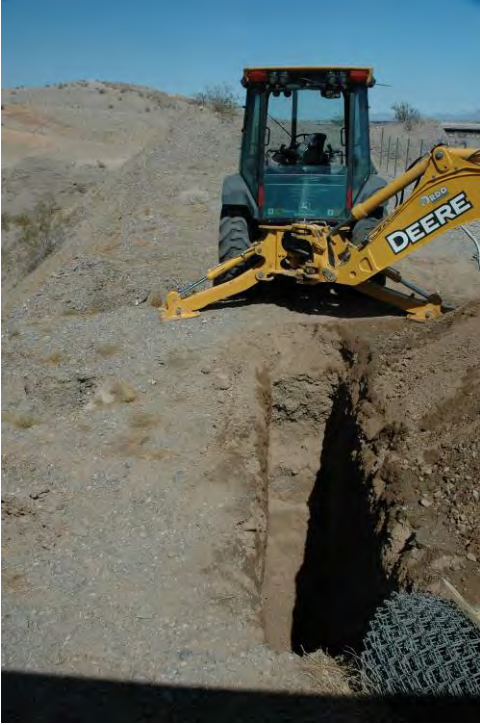
Photo 4: AOC12c-T1 west; east view
