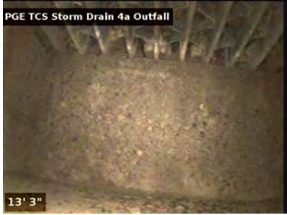
The catch basin was completely covered with debris at the time of the video.
