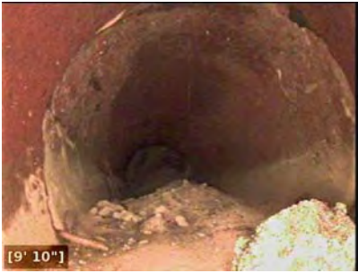
Dry sand and gravel in the bottom of the pipe. The distance from TD-3 is 178 feet.
