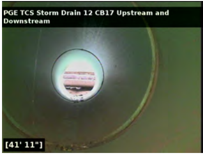
Trench Drain 2 ~4' ahead.
