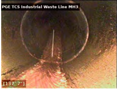
Subtle downward elbow, black steel pipe
