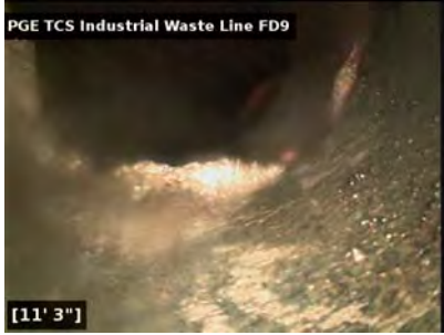
Grout intruding through red clay pipe joint
