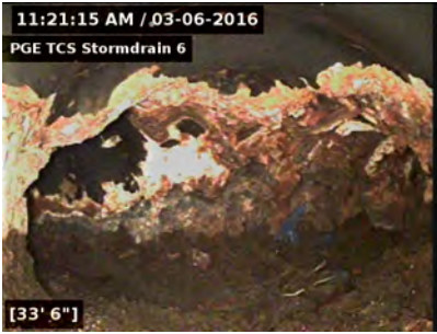
Photo of the "T" after we had flushed more water through the line.
