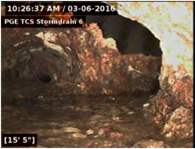
View of "T" looking upstream. Flow is coming from pipe on the right side of the photo, where we had added water to CB8. The camera was unable to proceed upstream to the left.
