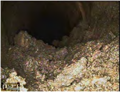
Debris in bottom of pipe.
