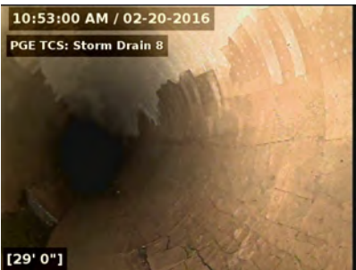
2/20/2016 10:53:00 AM Small cracks or scale in bottom of pipe.
