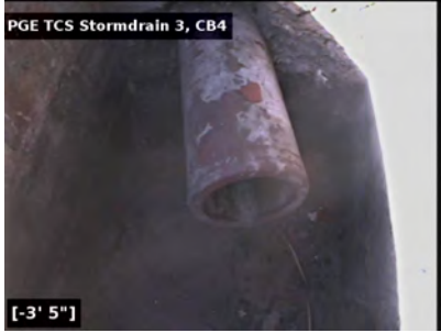
Catch Basin 3, looking at the outfall from the line that runs from CB4 to CB3.
