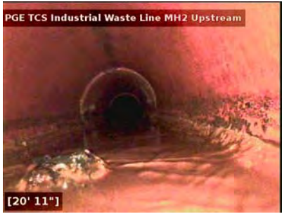
Debris and sludge in the pipe
