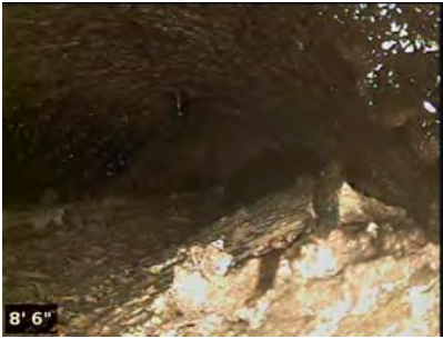
Debris in pipe.
