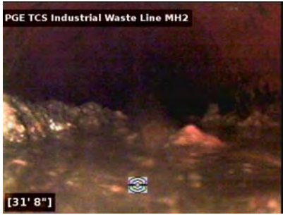
Heavy sludge build up and back flow. Appears to be red clay pipe.
