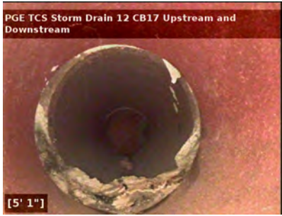
Clay pipe with grout intruding into pipe.
