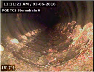
Steel corrugated pipe.
