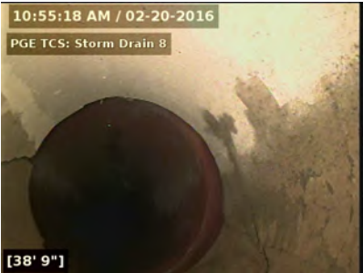
2/20/2016 10:55:19 AM Transition back to red clay pipe and elbow to the left, north and down slope.
