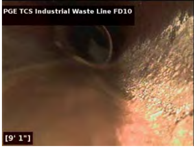
Elbow that enters the main line
