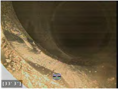
"T" fitting for the CB-21 line, on the left side.
