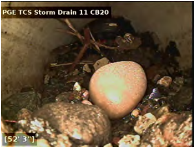
Rock and gravel blockage.
