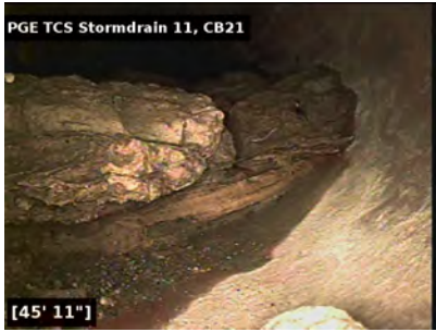
Debris in pipe
