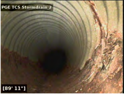
Corroded steel pipe with possible holes on the right side of photo.
