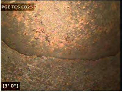
PG&E Topock Compressor Station
