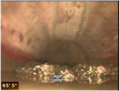
Standing water and some debris.
