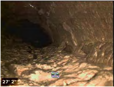
Debris in the pipe.
