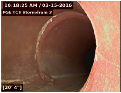
PG&E Topock Compressor Station
