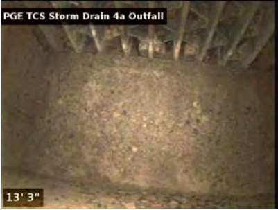
The catch basin was completely covered with debris at the time of the video.
