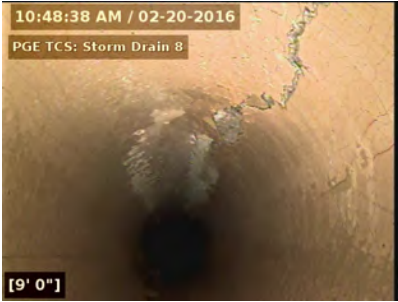
2/20/2016 10:48:38 AM Cracks present in top of pipe.
