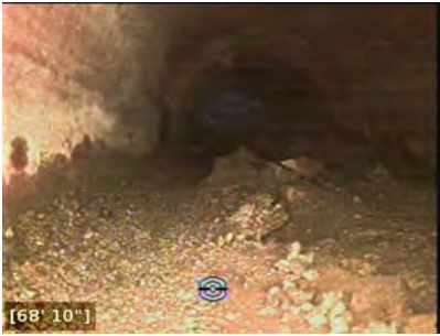
CB-22 in the far background. Debris in the pipe. Pipe is red clay, 8" diameter.
