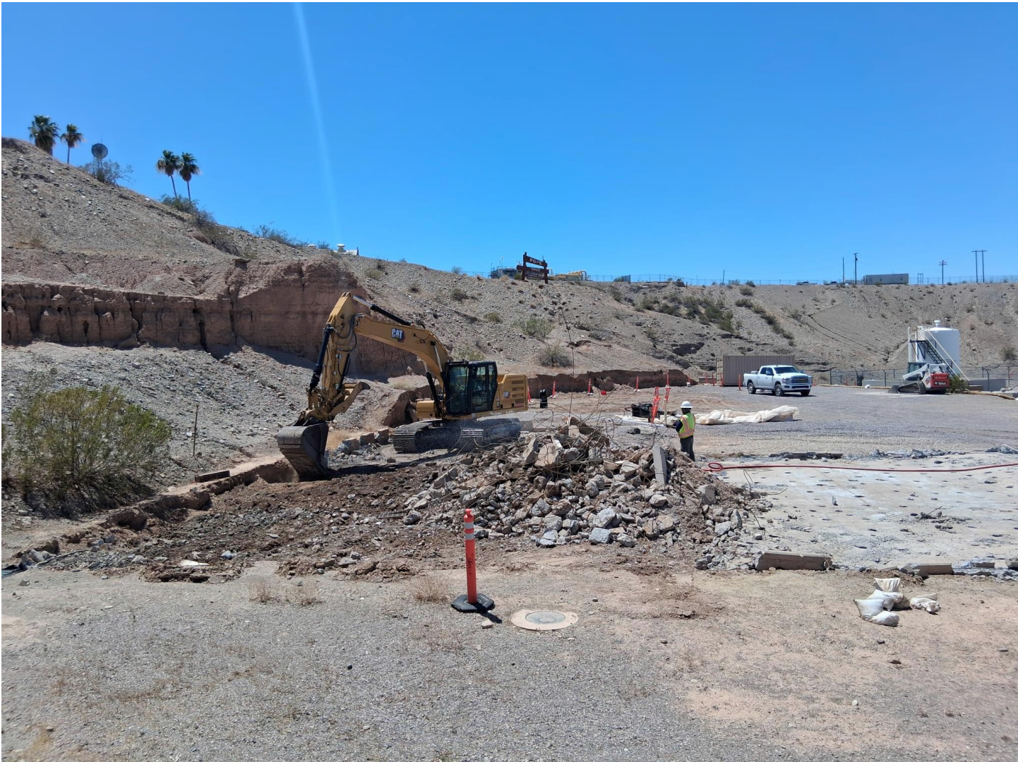
Photo showing the removal of the decon pad at the Transwestern Bench.
