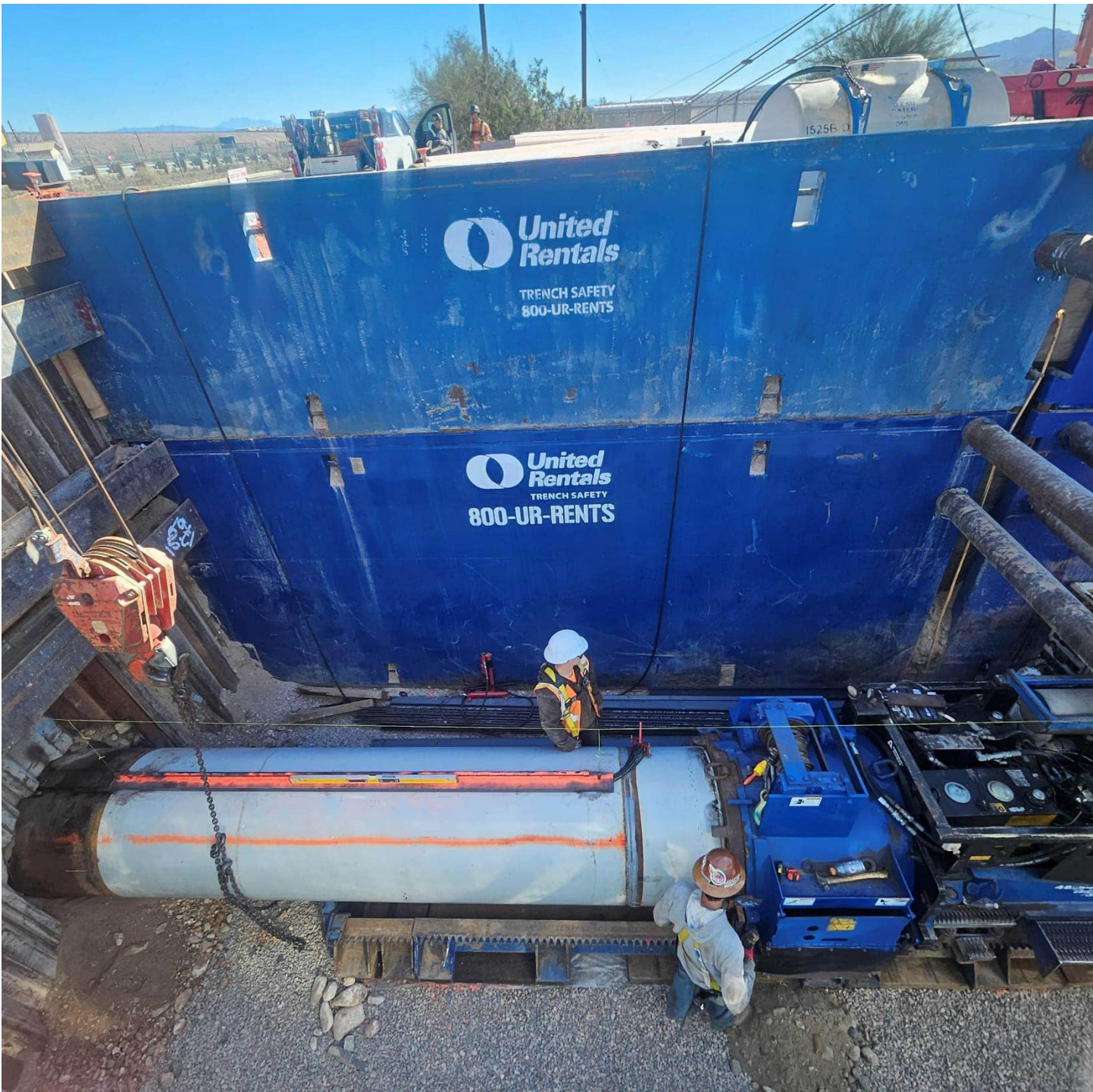
Photo showing a steel casing section with auger installed inside, being pushed under I-40.
