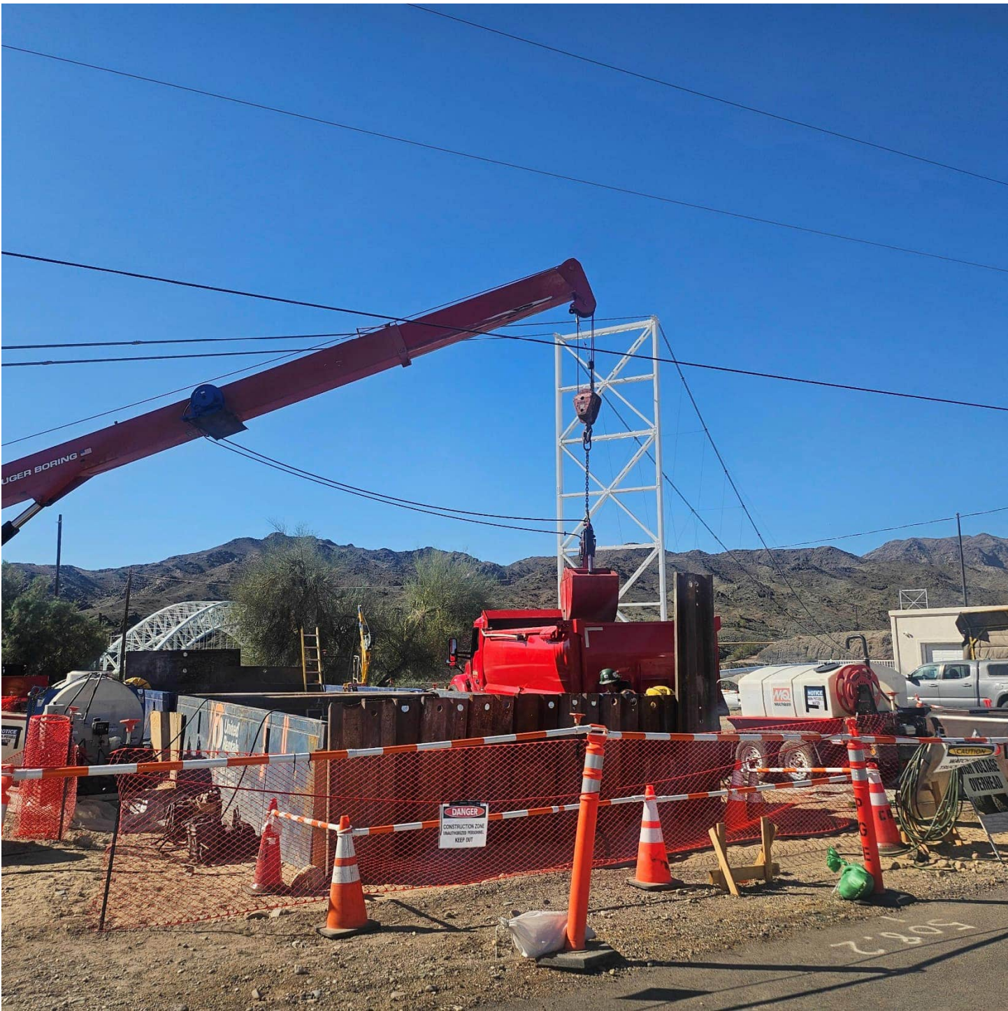
Photo showing a hoisted scoop bucket with excavated soil from augering under I-40.
