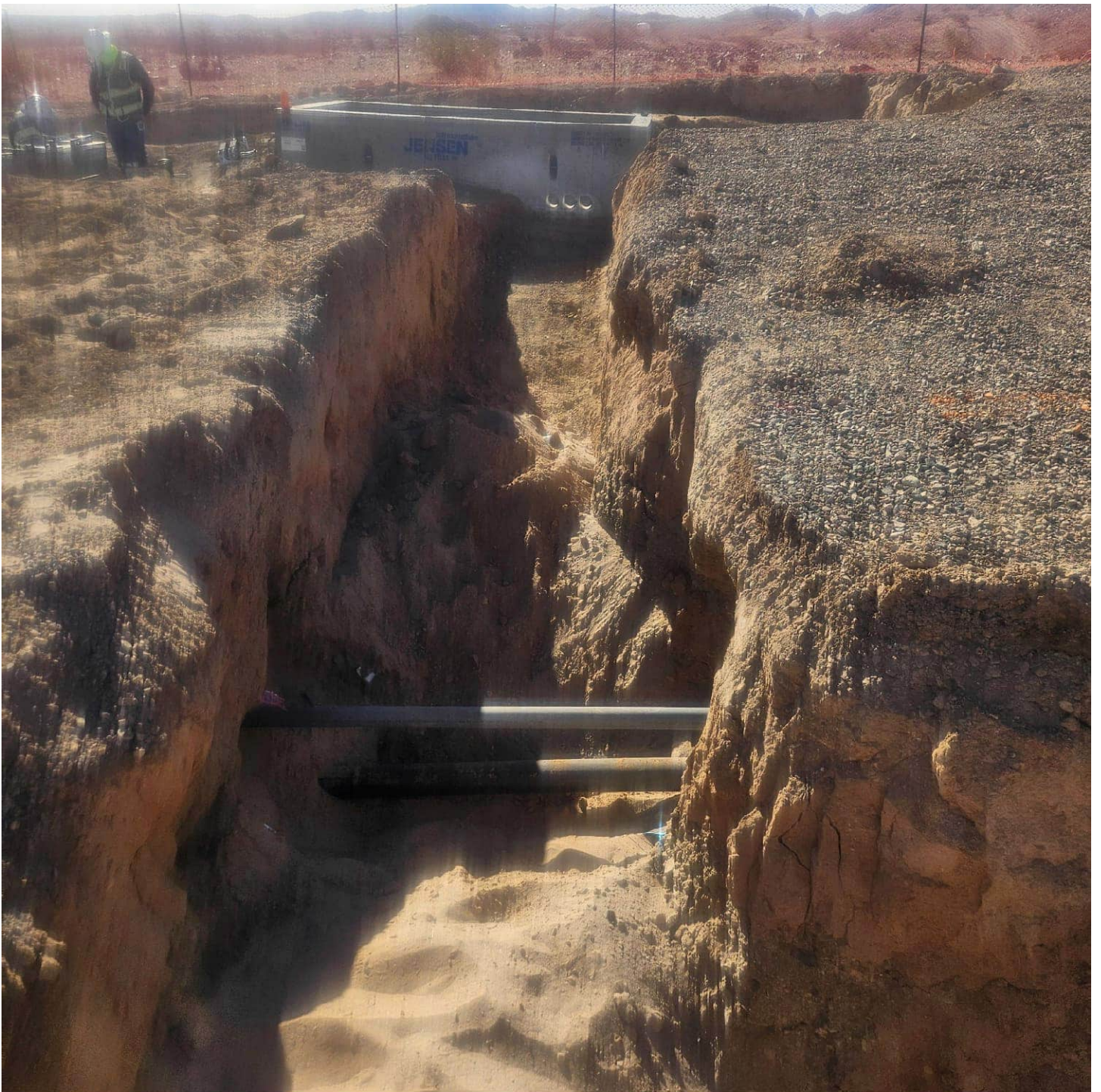
Photo showing Pipeline A trench near FW-01. Due to conflict with Pipeline A and with DTSC's approval, the IM3 pipe and conduit (shown in the foreground) were removed and stored within the IM3 plant fence line.
