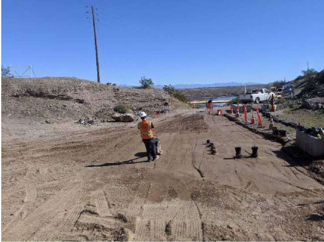
Photo showing earth fill compaction at the junction of Pipeline B and J.
