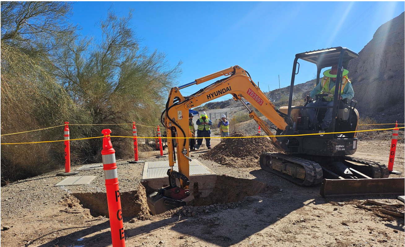
Photo showing trenching at IRZ-39 for the installation of belowground conduits and aboveground infrastructure.
