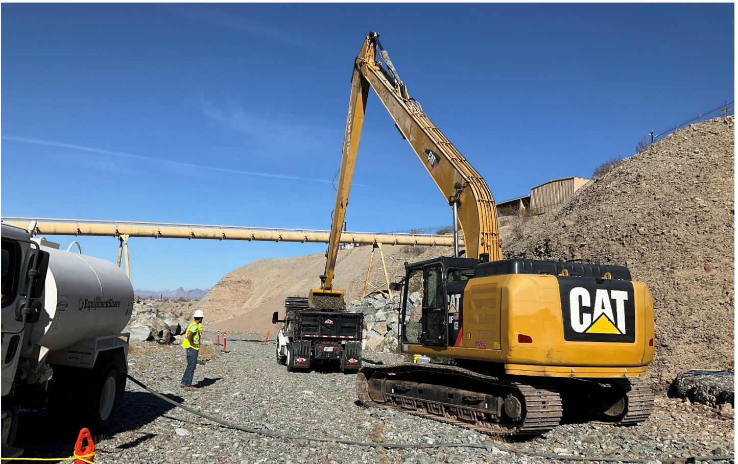
Photo showing the long reach excavator loading excavated soil/sediment into a dump truck.
