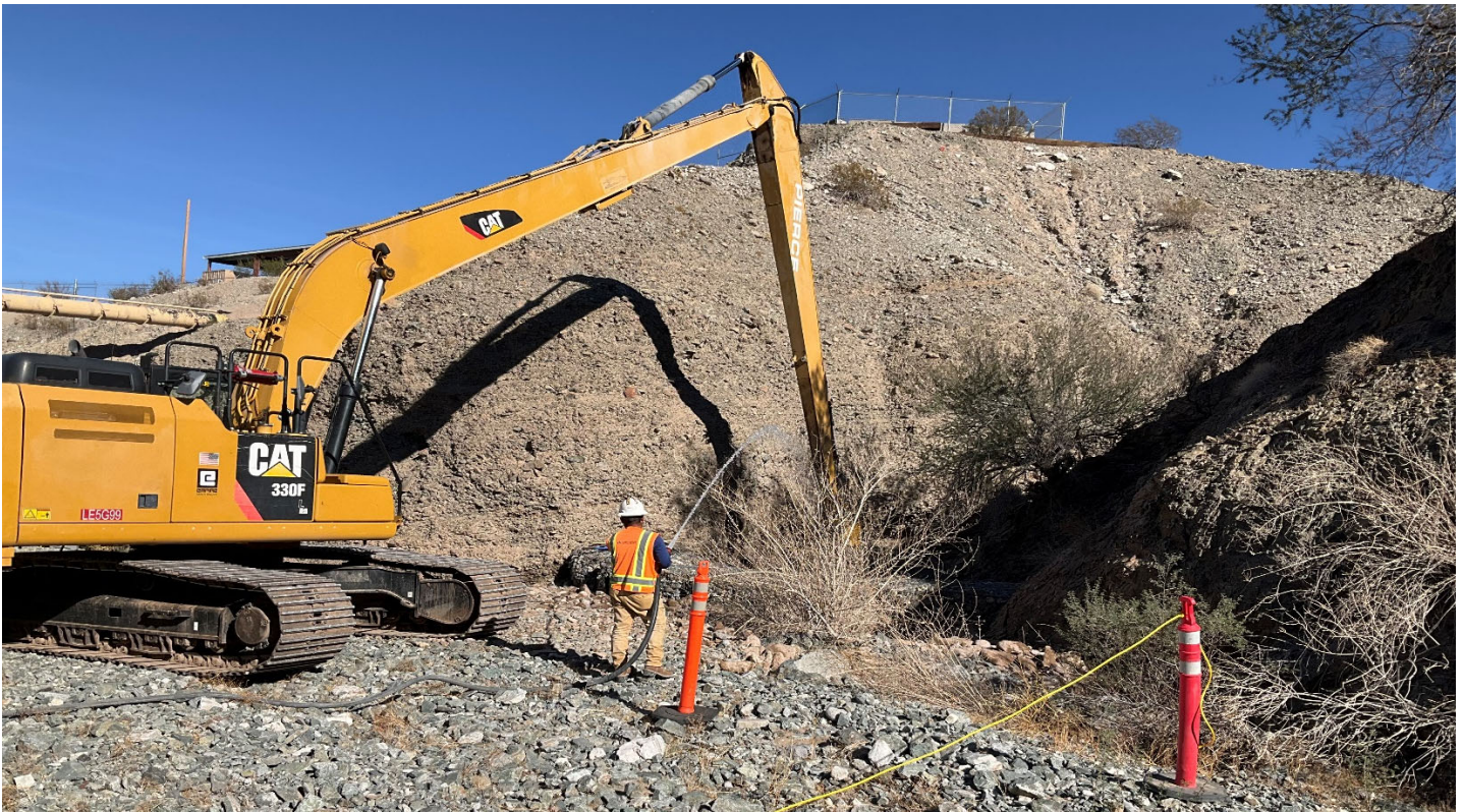
Photo showing the long reach excavator removing soil/sediment behind the AOC4 gabions in Bat Cave Wash.
