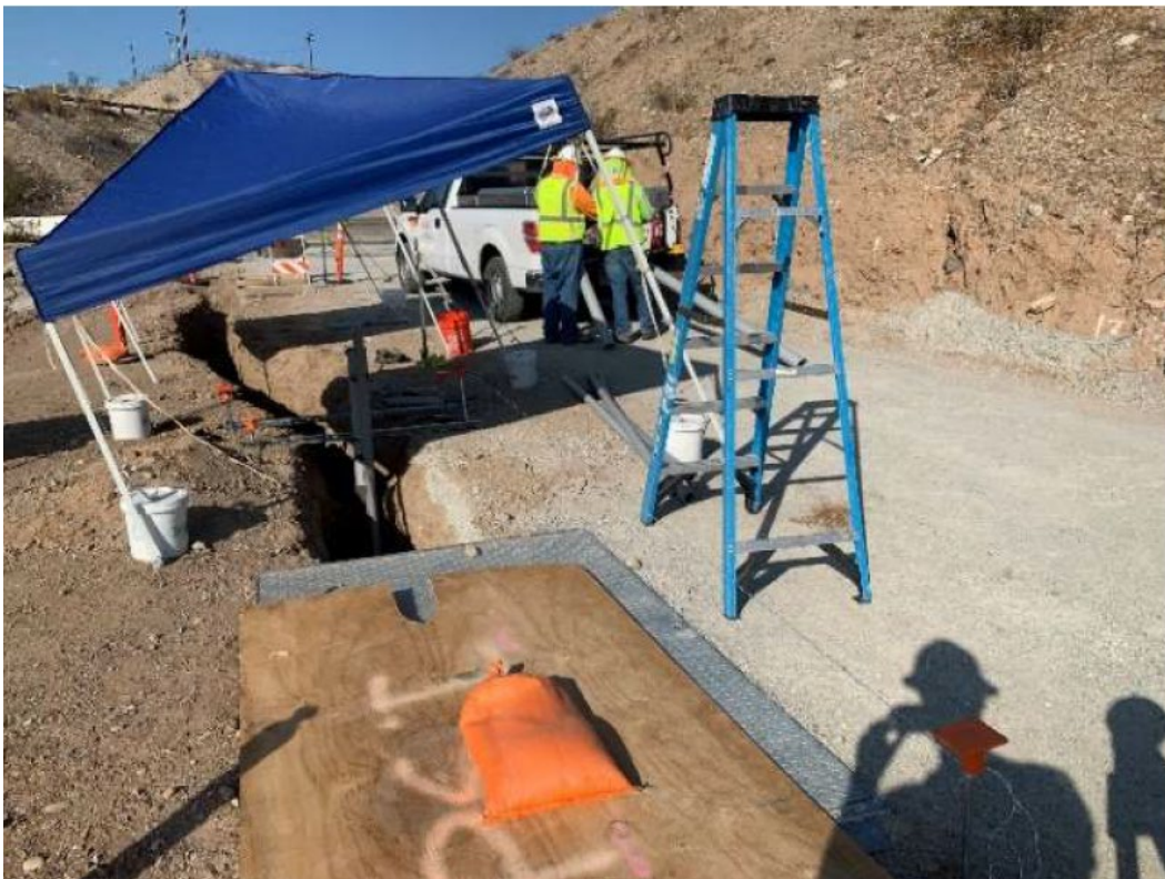
Photo showing transformer pad installation at Electrical Node 2 (Looking west towards TCS).
