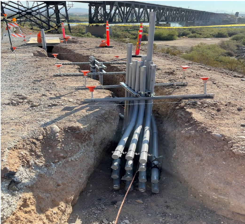
Photo showing conduit installation at Electrical Node 2 (Looking east towards the river).
