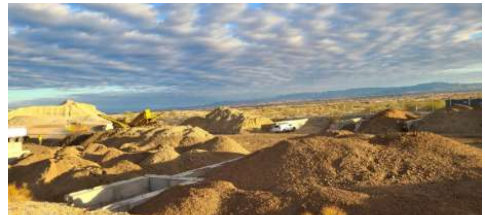
Photograph 3: Soil Processing Yard - more than 12,600 cubic yards of excess soil was generated during Phase 1 construction, of which 90% was reused onsite
