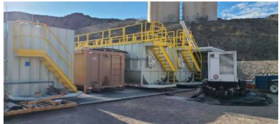
Photograph 2: Remedy Produced Water Conditioning System
