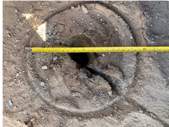
Core Depth: 0 to 0.5 Description: DR drill casing centered over pilot borehole. Date: 10/12/2022
