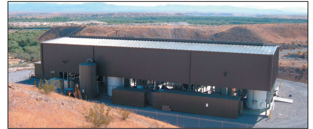
Treatment facility for Interim Measure No. 3
