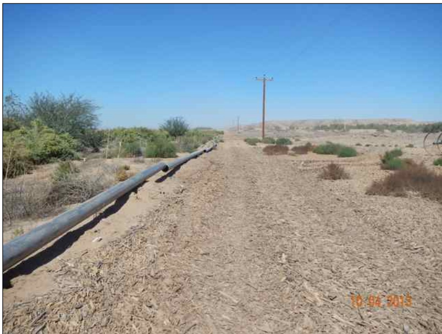
Photo 12. Irrigation pipe placed between HNWR-1A and Site B along existing power line right-of-way. Pipe was removed at project completion.
