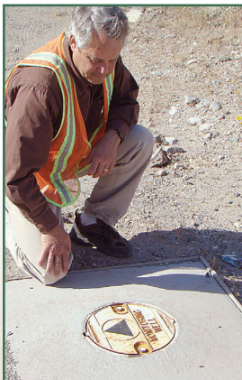
Pictured above is a flush mount groundwater monitoring well at the Site.
