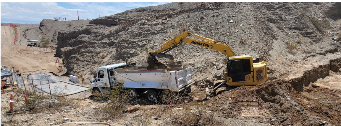
An excavator works to remove contaminated soil from federal land adjacent to compressor station property.
