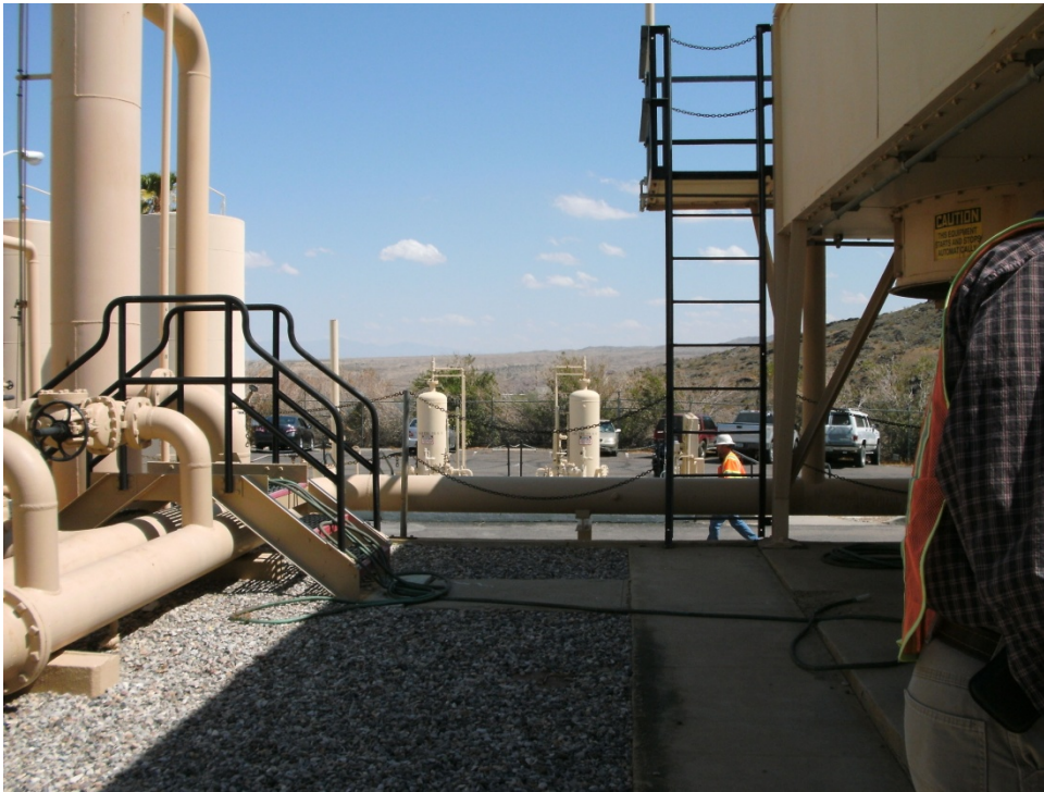
Photograph 17: AOC 15, Auxiliary Jacket Cooling Water Pumps, south side, looking east
