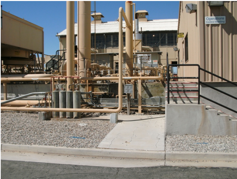
Photograph 22: AOC 15, Auxiliary Jacket Cooling Water Pumps, east access, looking west
