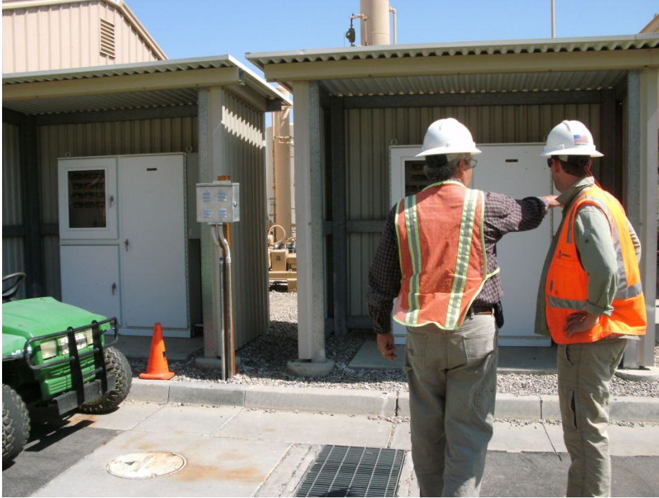
Photograph 21: SCADA cabinets immediately west of AOC 15, Auxiliary Jacket Cooling Water Pumps
