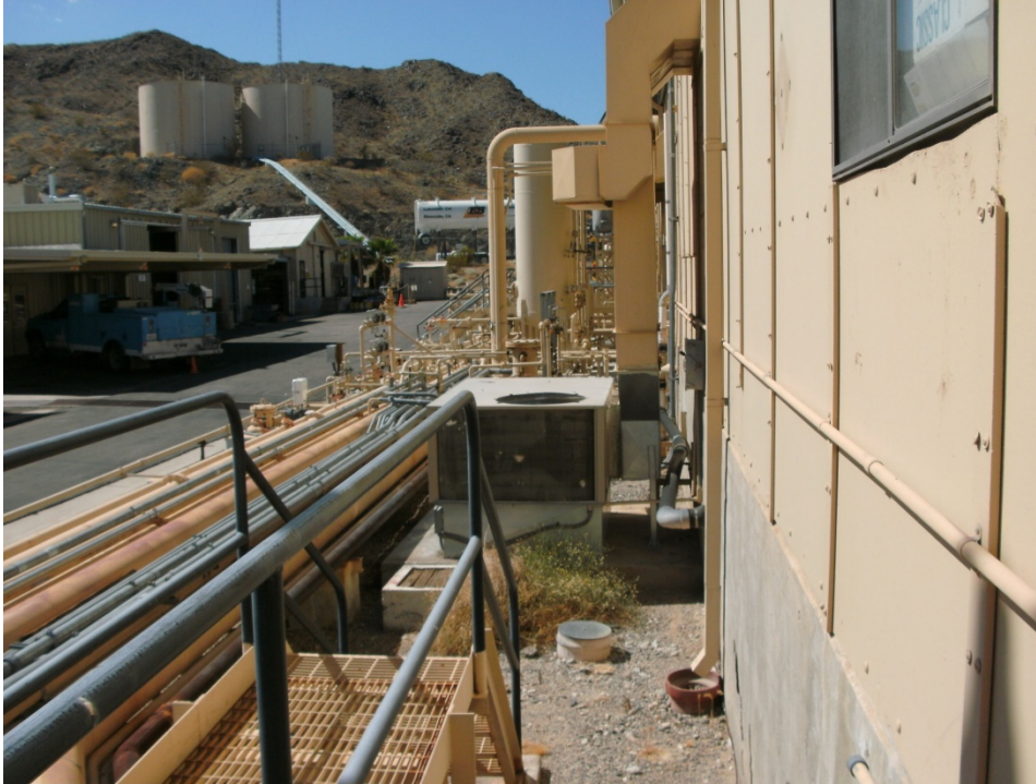
Photograph 53: AOC 25 Compressor and Generator Engine Basements, Auxiliary Building, east side, showing utilities, looking south
