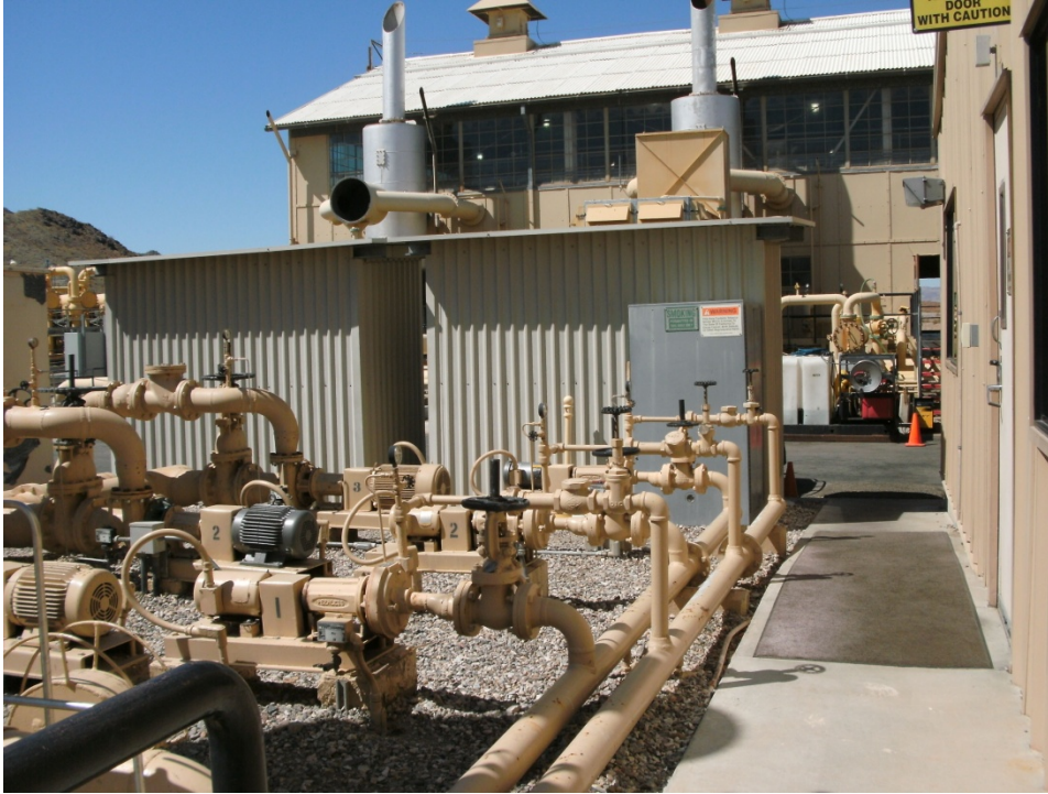
Photograph 23: AOC 15, Auxiliary Jacket Cooling Water Pumps, looking west
