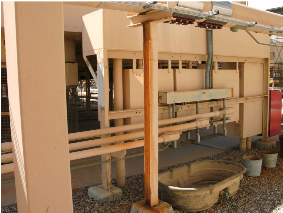
Photograph 40: AOC 19, Former Cooling Liquid Mixing Area and Former Hotwell, south side, looking west-southwest toward south Jacket Cooler Control Panel
