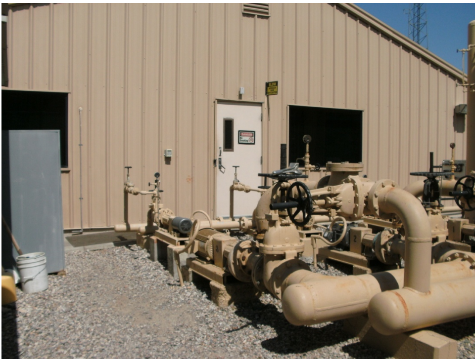
Photograph 18: AOC 15, Auxiliary Jacket Cooling Water Pumps, looking north to Control Building
