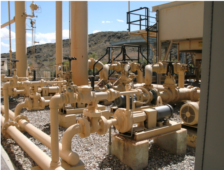
Photograph 24: AOC 15, Auxiliary Jacket Cooling Water Pumps, looking southeast
