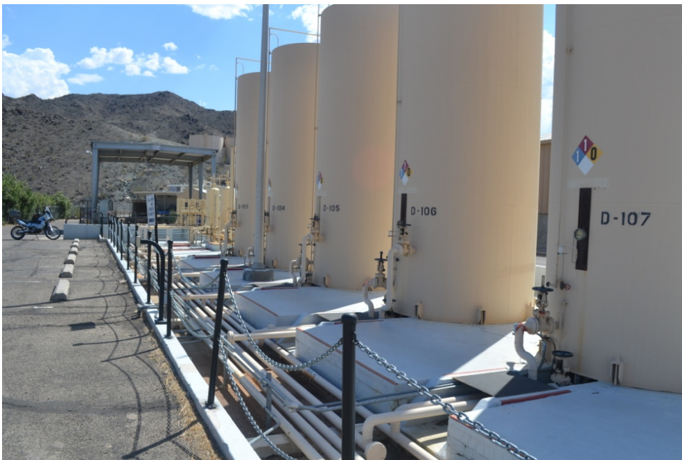
Photograph 66: AOC 32 Oil Storage Tanks and Waste Oil Sump, looking south along east side of oil storage tank area
