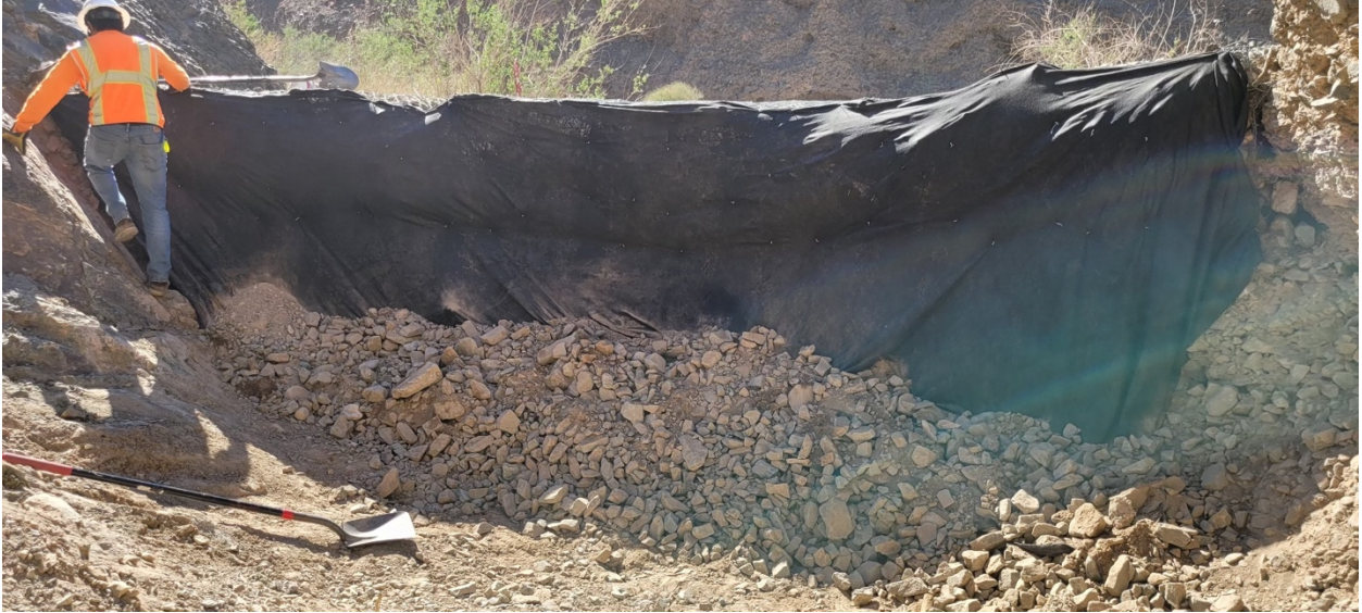
AOC 4 Gabion: Installation of Felt Fabric on Upstream Side of Gabion, September 21, 2021
