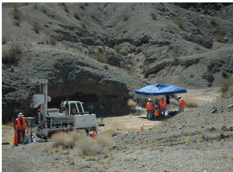
Soil sampling event at the Site in 2008. Soil sample collection in a ravine using a track mounted drilling rig.
